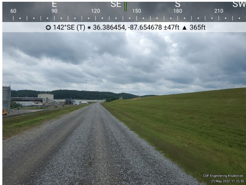
Photo D-2 View of northern dike of the Gypsum Storage Area. General conditions, no deficiencies observed.
