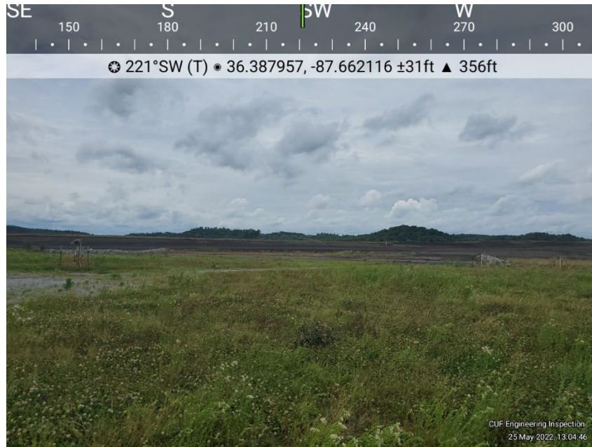
Photo E-3 View of interim covered interior portion of the Dry Ash Stack. General conditions, no deficiencies observed.
