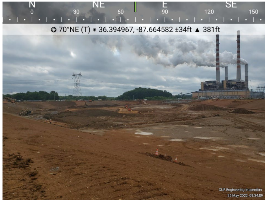
Photo B-2 View of the Stilling Pond (including Retention Pond). General conditions, no deficiencies observed.
