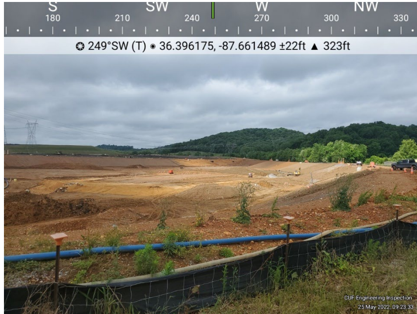
Photo B-1 View of the Stilling Pond (including Retention Pond). General conditions, no deficiencies observed.
