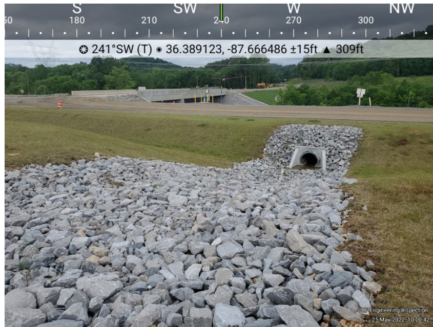
Photo E-4 Drainage feature connecting to perimeter road west of the Dry Ash Stack. General conditions, no deficiencies observed.
