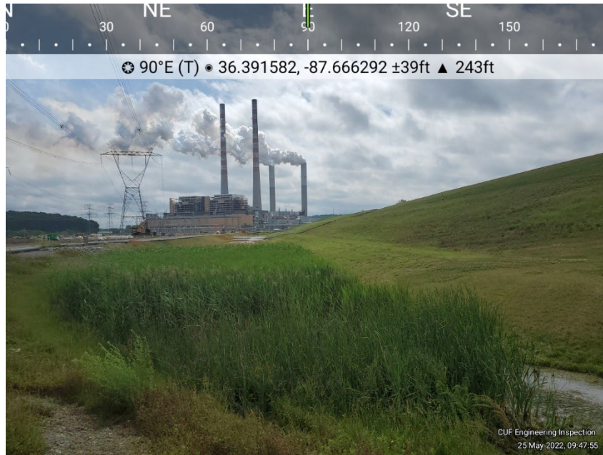
Photo E-2 View of the northern perimeter ditch at the toe of the Dry Ash Stack. General conditions, no deficiencies observed.
