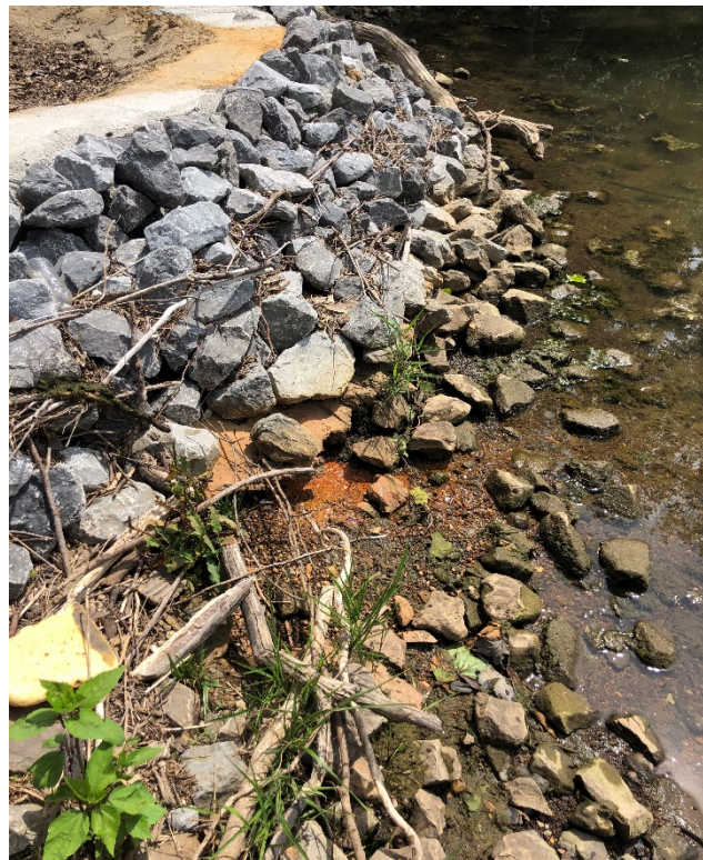
Photo 6 Seep 13 at Ash Pond E on May 27, 2021 to show observed seepage. This area could not be viewed during the Annual Inspection due to the elevated river level.
